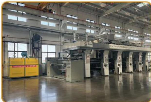
江苏复合机供热 Tiangsu compound machine heating
