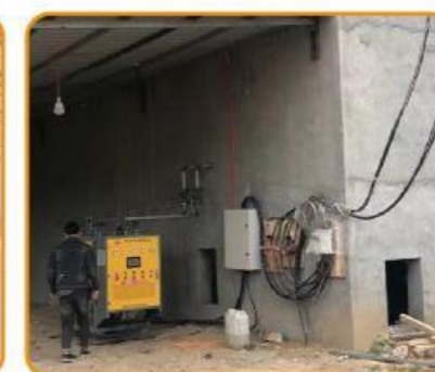
东北电加热带烘房 Northeast electric heating belt drying room
